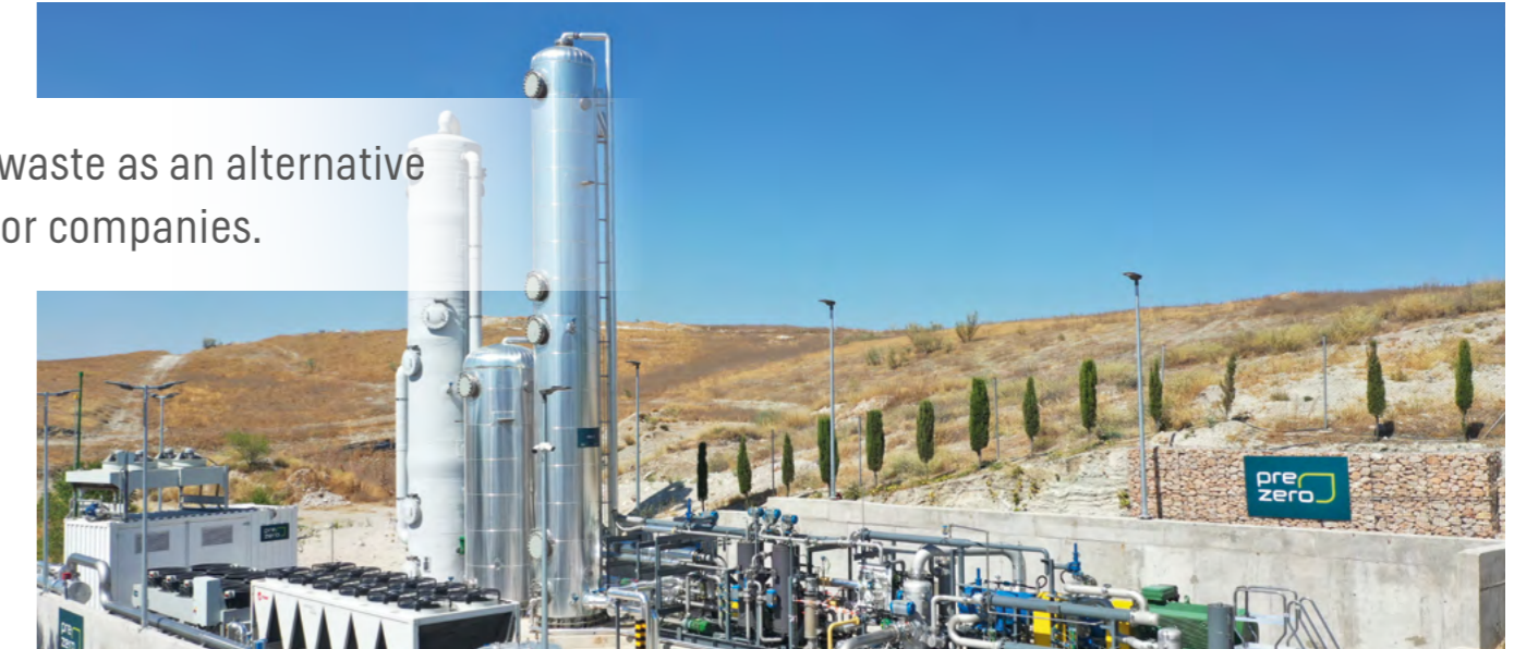
The Valdemingómez biogas plant processes the organic waste of the 3.2 million Madrid inhabitants.
